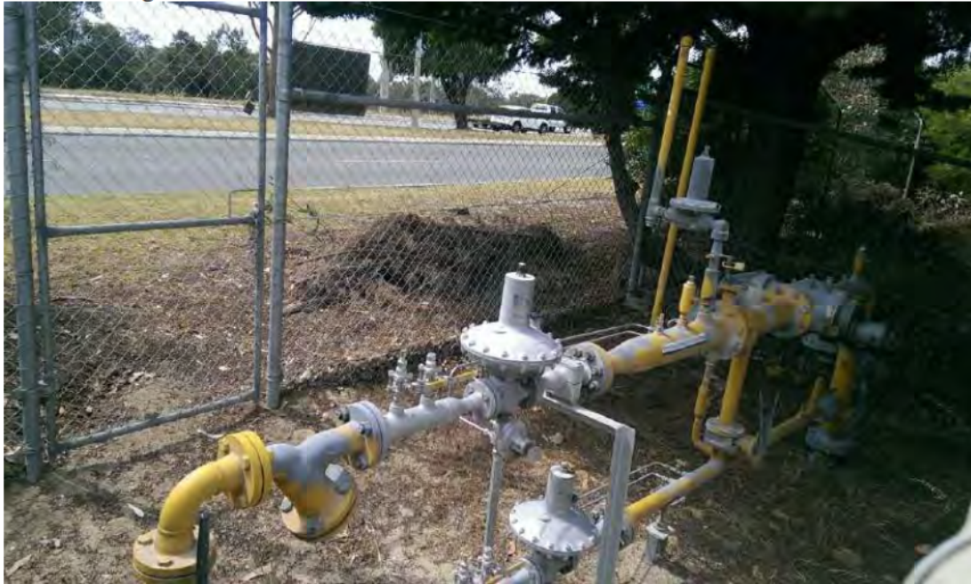
Figure 10 - Existing Gas Meter Set
