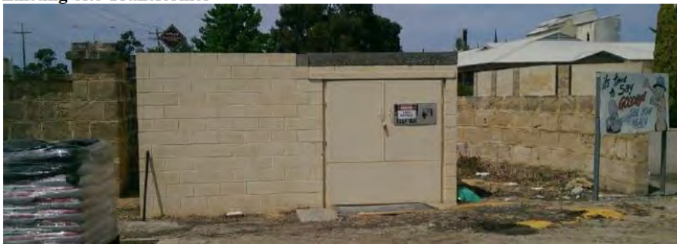
Figure 9 - Existing Site Transformer
