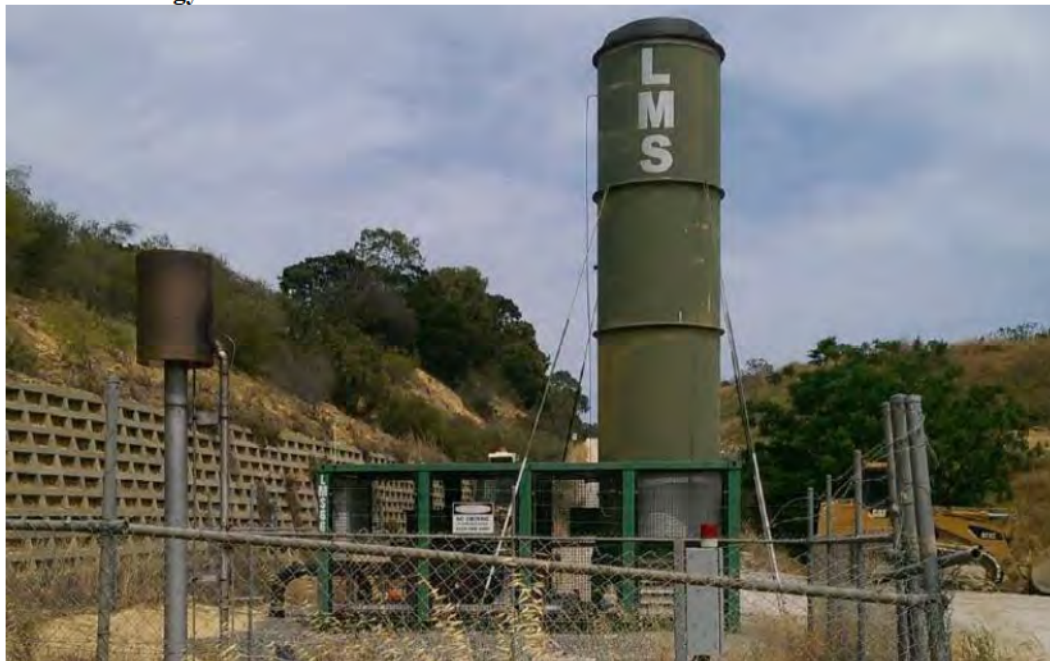
Figure 8 – LMS Energy - Methane Burn Towers
